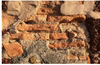
Figure 5: Later mortar for brick structure
